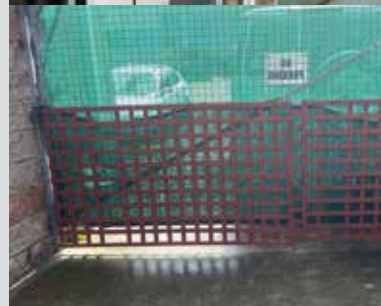
Gate rusted and dangerous. Lattice was added to the bottom to stop the playgroup escapees and protect from any possible injury
